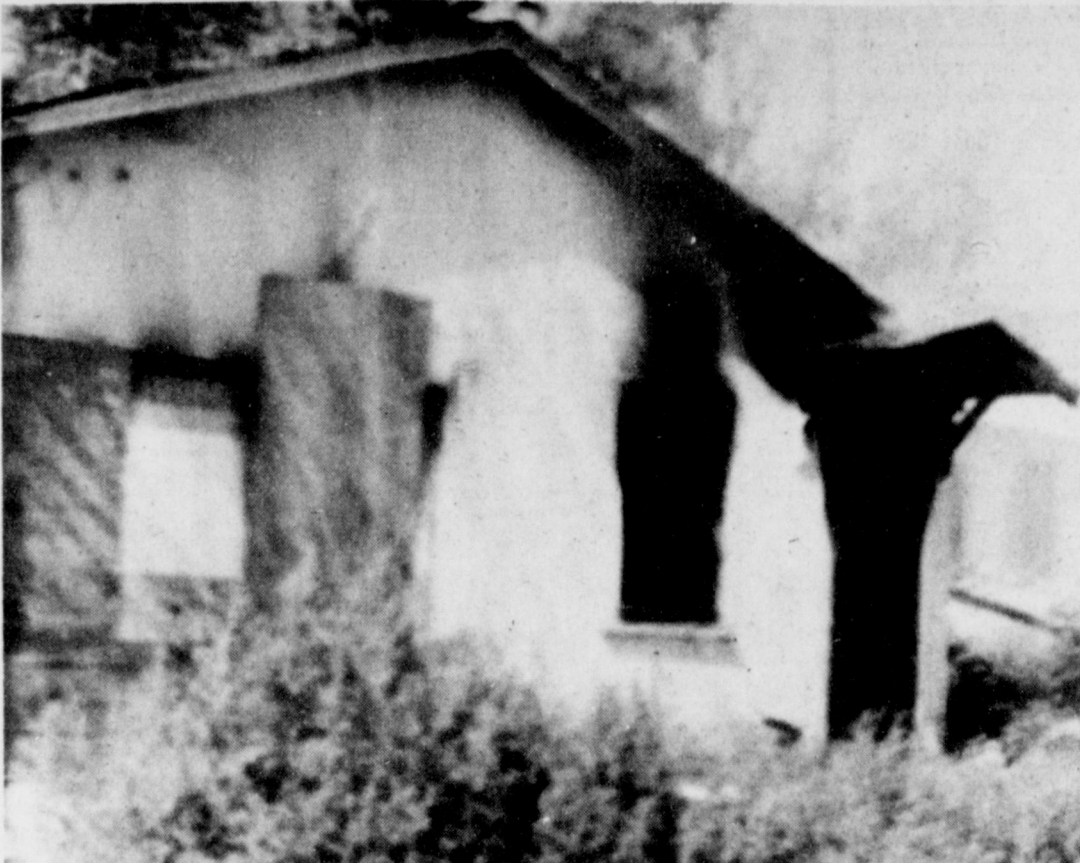
FIRE DAMAGES HOUSE . . . A fire broke out late Saturday morning in this house in the 500 block of West Avenue B. Dense smoke partially obscures the unoccupied house shortly before firemen arrived. Heavy damage done to the front part of the partially boarded up home which was used to store carpenter tools. Cause of the fire has been undetermined.
