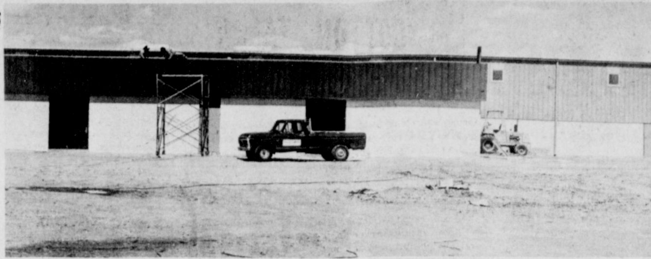
CIVIC CENTER CONSTRUCTION--Still continuing is construction of the Bailey County Civic Center and Coliseum. Workmen were busy Monday afternoon with the roof of the front portion of the building. It is not expected to be ready for occupancy until late May or in June.
