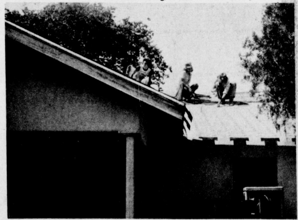
STORM DAMAGES HOUSE --A mile south and just over a mile west of Needmore, roofers attempt to get a roof back onto a house on the Loyd Davenport farm. Prior to Monday night's more than two inches of rain, the shingles had been removed for a new roof. The inside of the house was inundated, damaging everything in the interior of the home.
