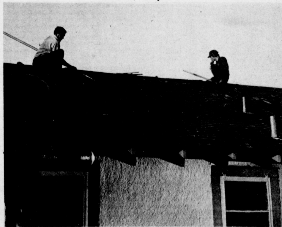
TEARING THE ROOF OFF...Two Muleshoe Volunteer Firemen are shown with hooks tearing cedar shingles off a house at Progress which partially burned Sunday morning. Firemen blamed a water heater in the bathroom for the fire which left heavy damage to the bathroom, one bedroom, ceilings and the roof of the home.
