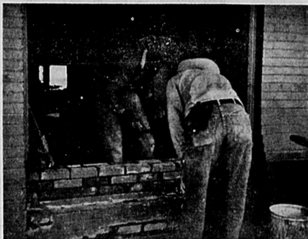
The Baird Star — Getting a face lifting this week after a pickup truck ran into the front of the building some three weeks ago. Here you see workmen, W. A. (Slim) Robbins and Alva Dawkins, repairing the damage. Facelifting plans also include painting the front of the building.
