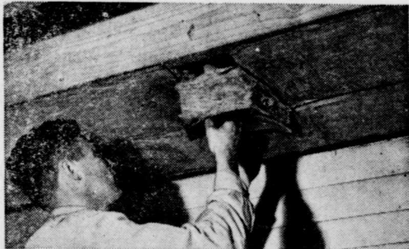
Workman carefully fits section of 6-inch mineral wool batt into place between two adjacent batts to give full, gap-free protection in the ceiling of this house being insulated for air conditioning. This goes along with the advice of home building authority Andrew C. Lang, who says: "Insist on proper installation of insulation to get full value from air conditioning."
