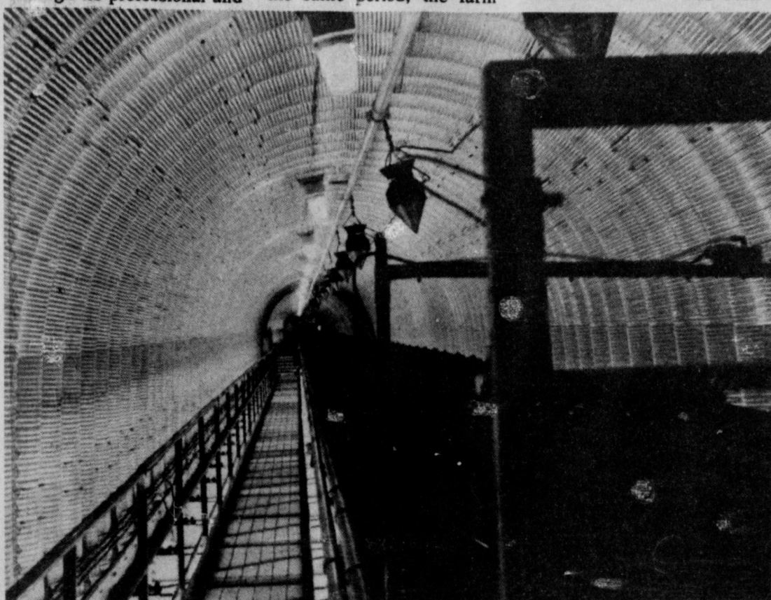
COAL CHUTES--The coal chutes which transfer the coal after it is dumped from the cars into the stockpiles awaiting grinding are dust-protected with water sprays, as the coal moves along the conveyor. This photo shows the inside of one of the two coal chutes at the Roy Tolk Plant.
