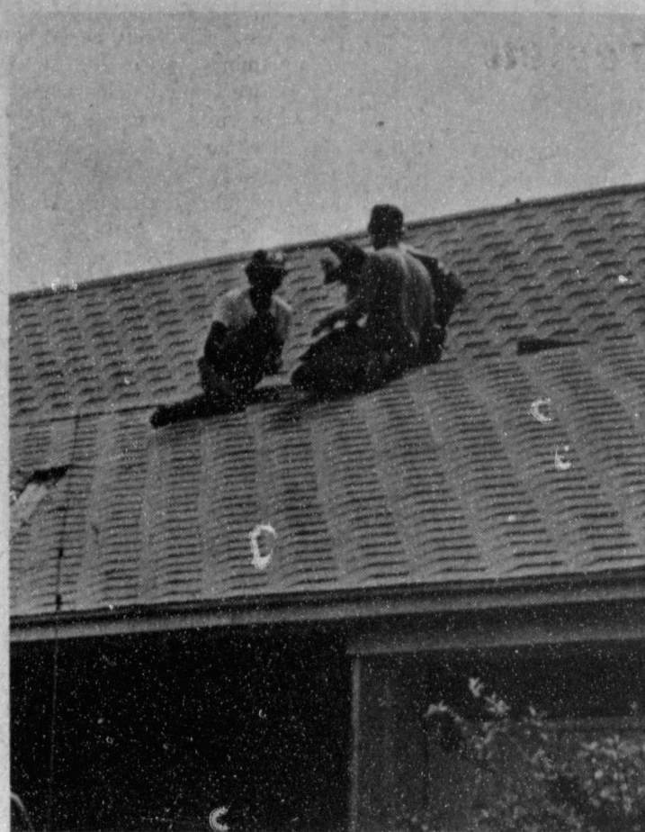
ROOFING REPAIRS --Many local and area buildings and homes are being repaired from the past month's hail damages. This scene depicted above is one that is commonplace in our city at this time.
