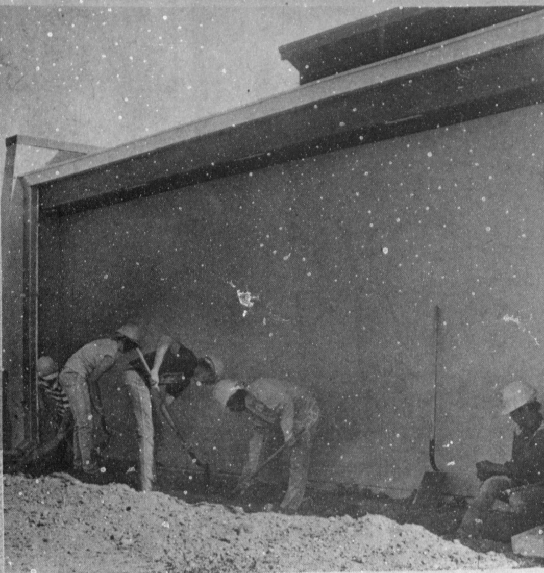
YCC — BUILDING A FUTURE AT THE REFUGE — Busy building a foundation for a retaining wall at the office building were these members of the Youth Conservation Corp. They are in an eight week program of renovation at the Refuge and will be busy each day, five days a week, as they renew and rebuilt and re-paint at the Refuge.
