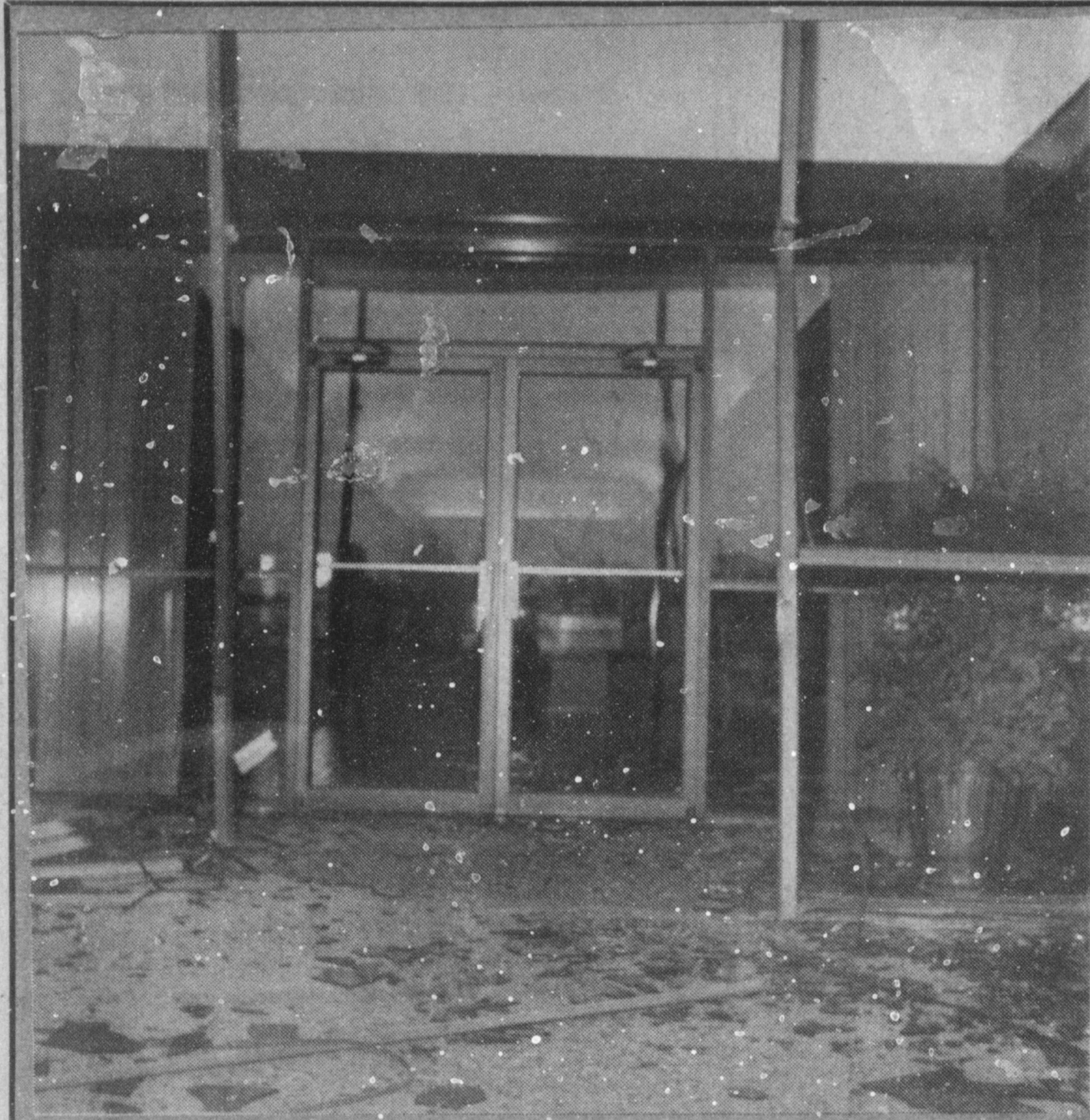
ANYONE FOR AN INSTANT DRIVE IN?—Muleshoe State Bank was rather surprisingly, turned into an 'instant drive in' early Tuesday morning, when an unknown individual or individuals, drove a vehicle through the first set of doors on the west side of the bank. They then deposited the doors nearly a block south in an intersection and left. Muleshoe City Police Department officers were investigating the criminal mischief at presstime. No one had been taken into custody.
