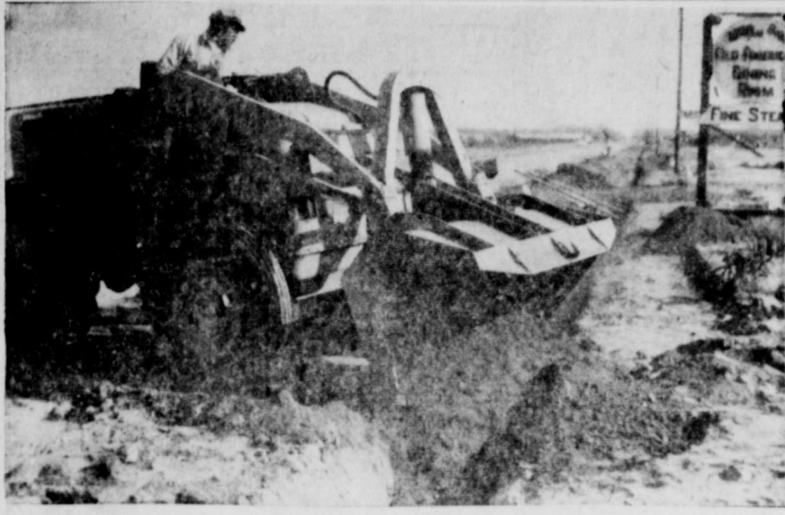
PIPE-LAYING OPERATIONS are well under way today for the 2 1-4 mile water main from Thirteenth Street west to the reservoir. (Advocate Photo)
