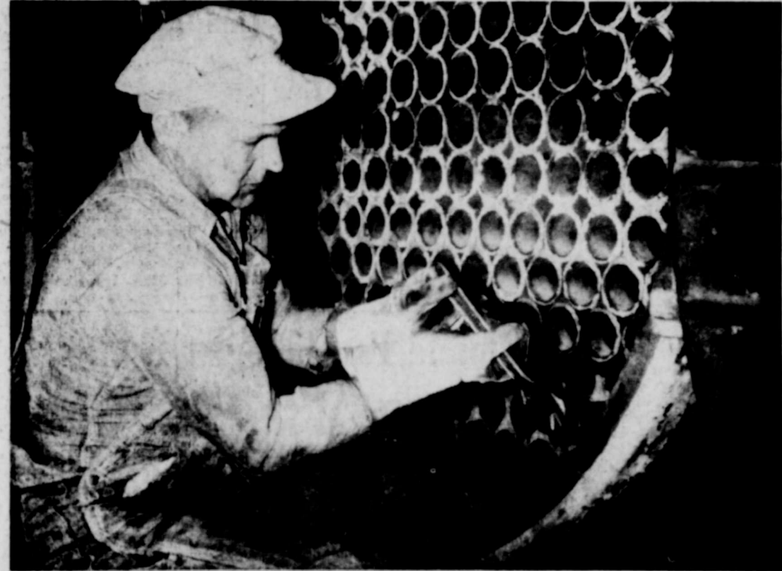
A LEAKY BOILER, that is delaying the opening of school at Junior High, is repaired by Tommy Bell, a boiler expert from the United States Potash Co. (Advocate Photo)
