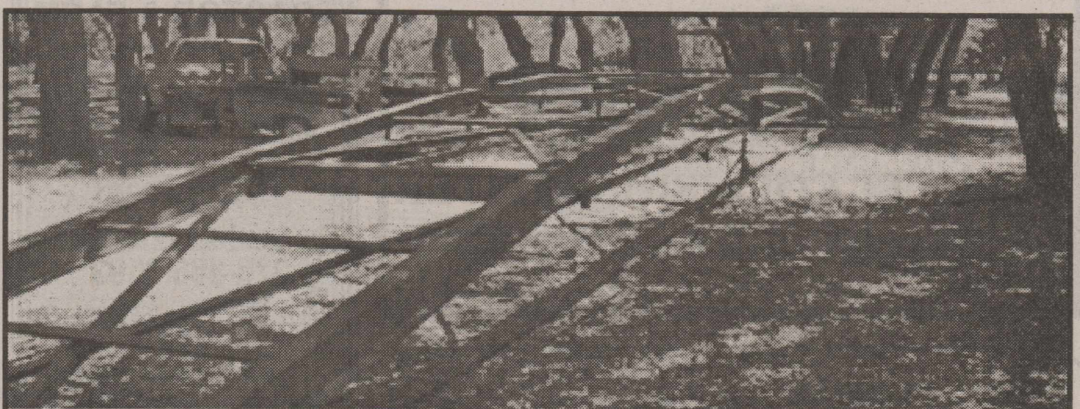
Turkey Creek Bridge — The Bridge Project is nearing completion. Rex Beggs has finished the welding on the bridge and plans to paint it are underway. Next week, the bridge should be moved to its final location and flooring will be installed. Once the floor is installed, only minor finishing touches will be needed to complete the project. Diligent efforts are being made to have the bridge completed in time for the Robert E. Howard Days.
