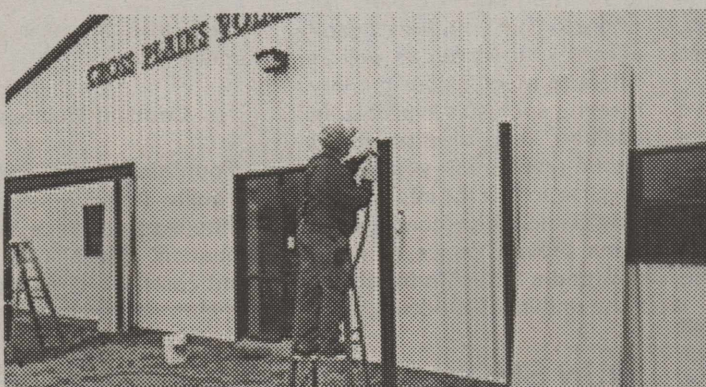
Fire Chief Rickey Carouth working on the front entrance of new firehouse
