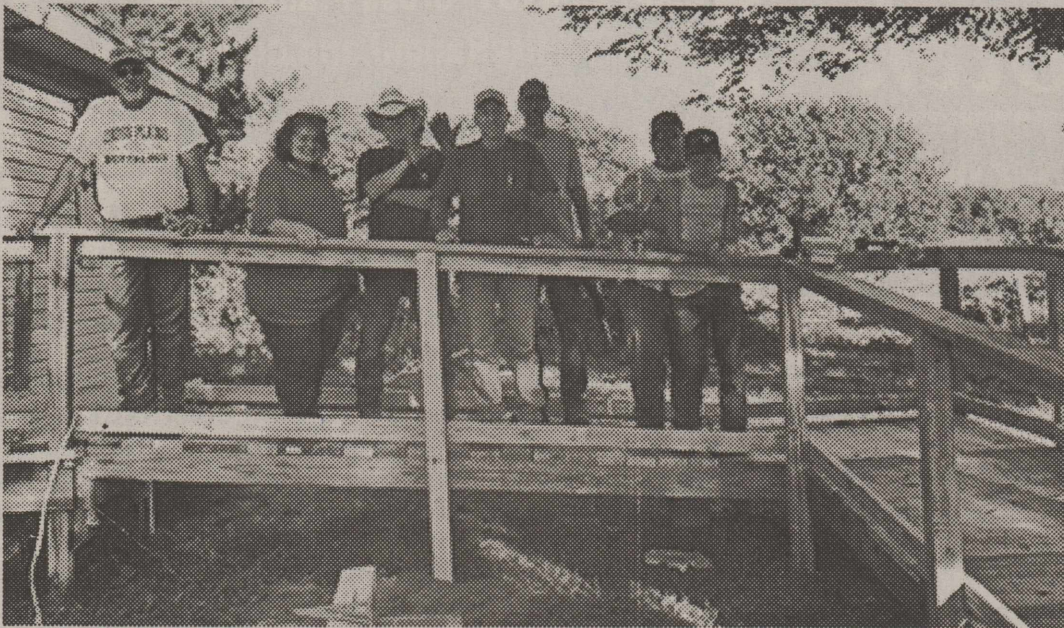
The Biggest Project - A 26 ft wheelchair ramp. Dozens of workers started at 8 a.m. and completed the huge job at 6 p.m.
