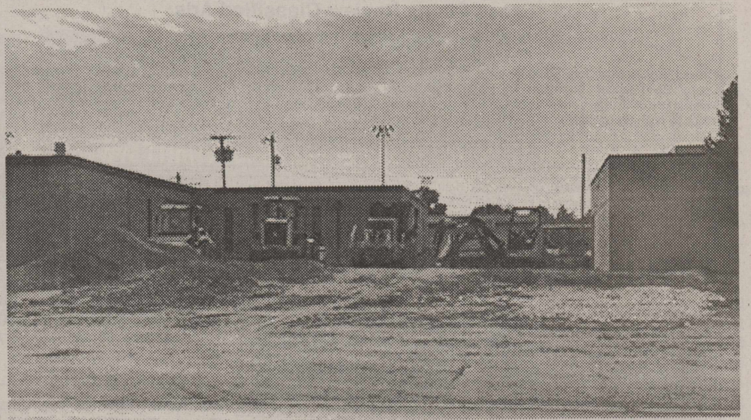
Building the New Band Hall -- Construction on the new band hall at CPISD. The demolition is done as the work enters the third week.
