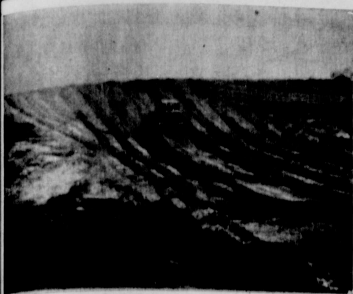
Pond being constructed on the Johnny Burson Ranch. The pond will furnish livestock water and better grazing distribution.
