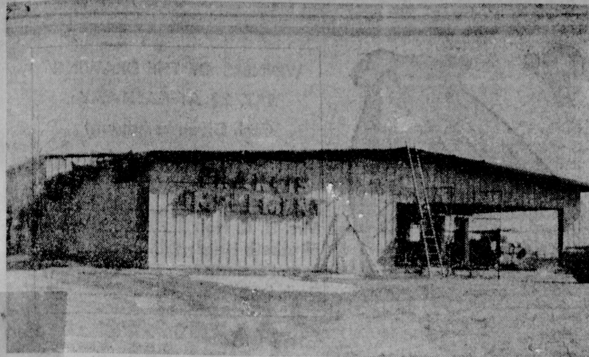
NEW CONSTRUCTION — New Home to be of Francis Implement nearing completion West of Muleshoe. The 7,200 square foot steel, pre-fab building will be completed about March 15th. It is being erected by B & C Builders, Inc.
