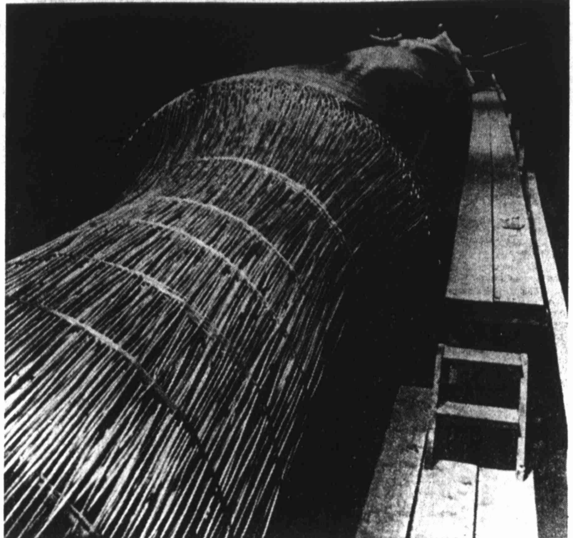
COLD WAVE—Aluminum, which becomes stronger rather than brittle in cryogenic (super-cold) applications, is scheduled to assist in the transportation of natural gas from Algeria to the United States. This photo shows a portion of the 330 miles of aluminum tubing used by a giant heat exchanger being fabricated by Air Products and Chemicals, Inc. Alcoa will supply 2,000 miles of coiled drawn tubing for six heat exchangers planned for importing gas. The gas will be liquefied and frozen for shipment by tankers.
