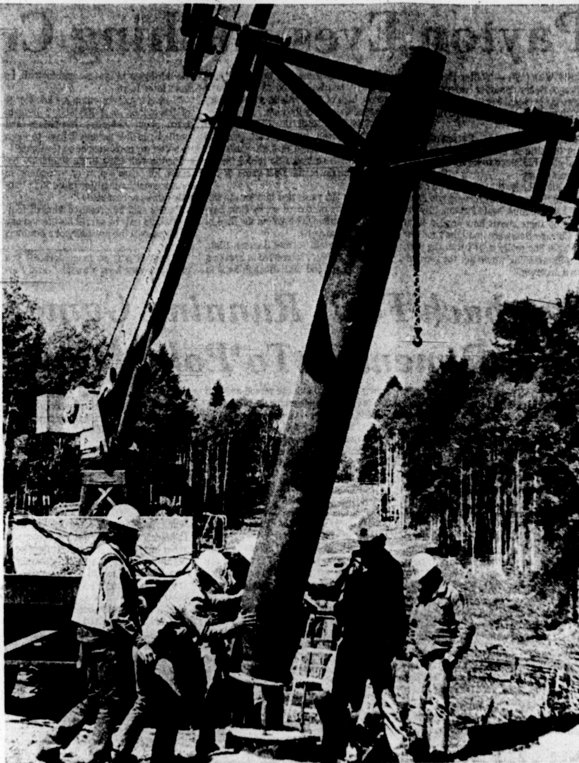
EASY DOES IT—A new double chairlift for skiers is being constructed at Red River, N.M. Dubbed the "Gold Chair" the 1,200-foot-long lift will have a capacity of 1,200 skiers per hour. The Red River Ski Area began making snow Oct. 16 in preparation for the upcoming season. The artificial snow will serve as a base for the first natural snowfall, assuring an early ski season.
