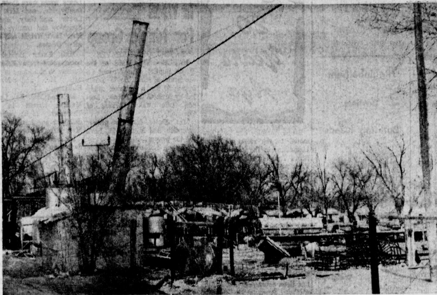
CANNERY GOES DOWN - Fading from the Muleshoe scene these days is the old Muleshoe Canning Co. plant on East Fourth. It is being razed by Morgan
