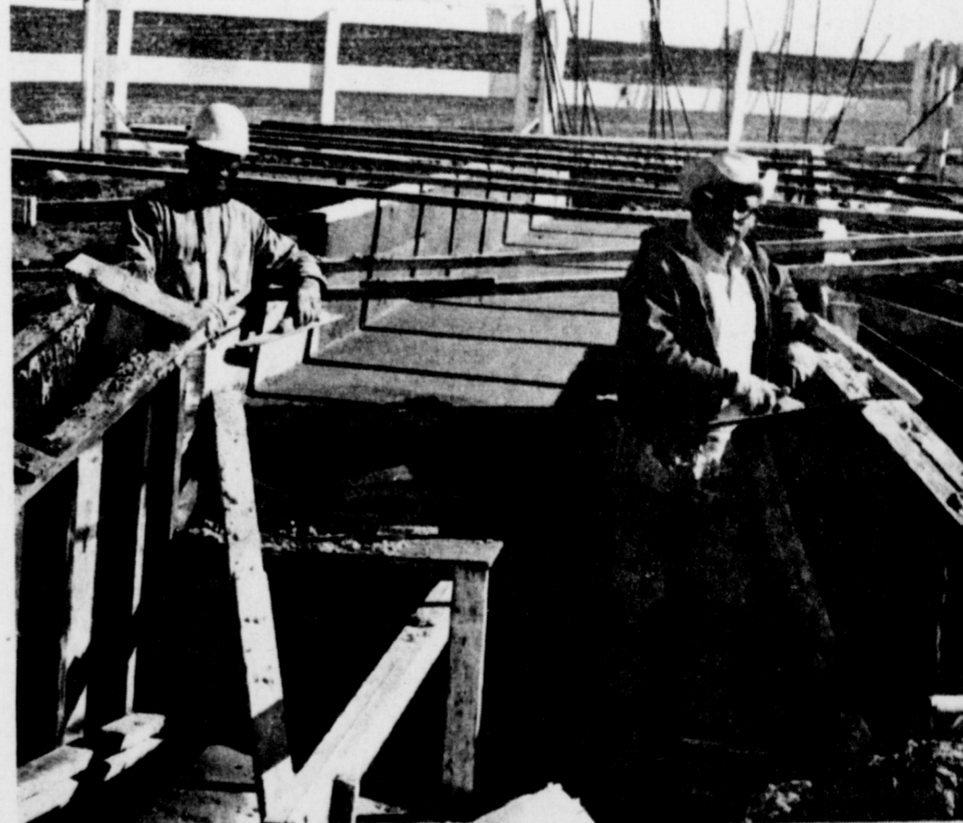
ROAD CONSTRUCTION UNDERWAY ... Construction is well underway this week on the Friona Highway. Construction plans are to widen Highway 214 from the Bailey County line to Friona. An overpass will also be constructed over the railroad tracks on the south side of Friona. This picture shows workers constructing a culvert just across the Bailey County line.
