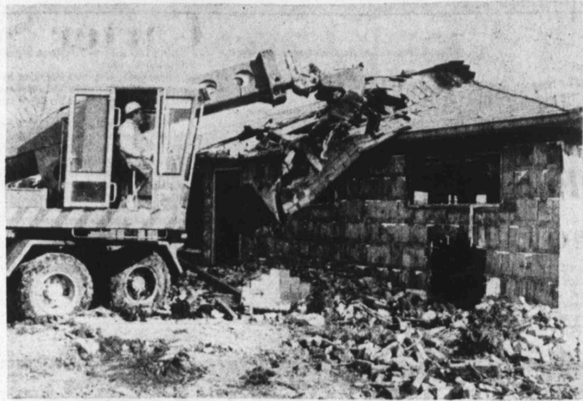
DEMOLITION BEGINS — Workmen Tuesday began taking apart the Norwood Park home of John Wayne Gacy Jr. after all appeals were overruled by the Illinois Supreme Court. Gacy
