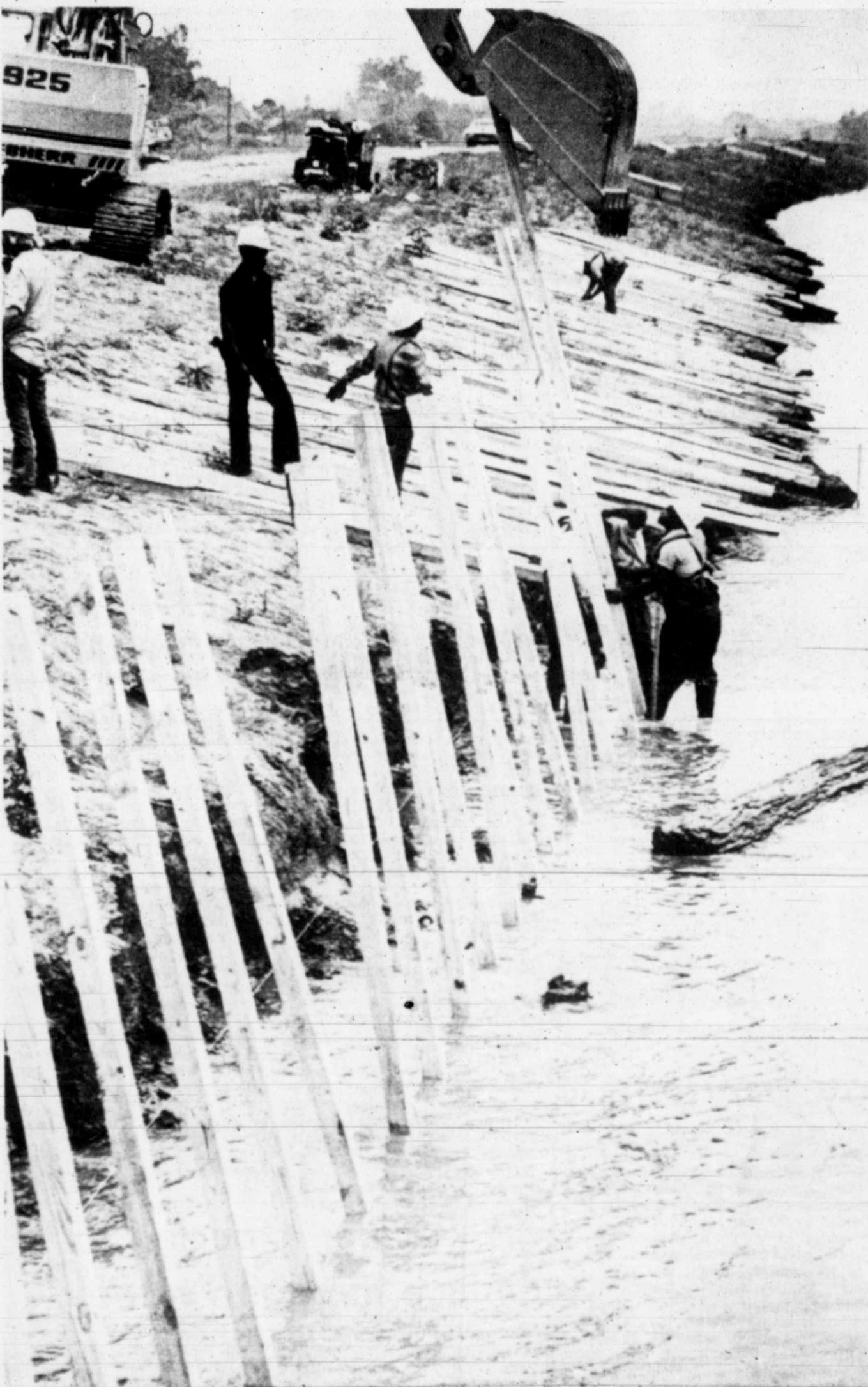
Workers spent the weekend erecting a board fence along a 1,900 foot section of the Mississippi River levee in Baton Rouge, La. The fence, intended to stop erosion of the levee by high water, will
