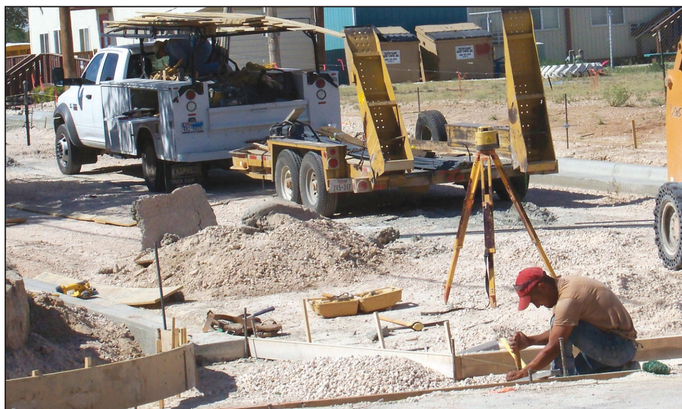
Work is underway on the CDBG paving project at Hickory and Houston.
