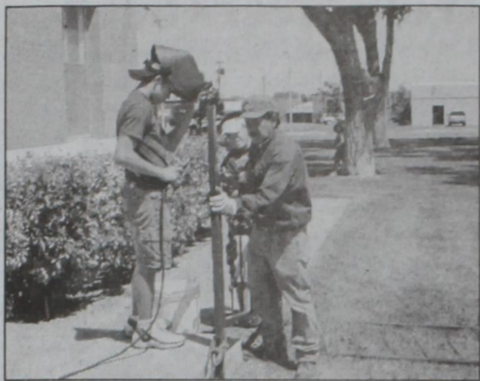
Journal photo: Beatrice Morin Arzola's Ornamental Iron recently installed handrails at the south side entrance of the courthouse. Pictured are (from left) John Michael Salinas, Israel Rodriguez and Victor Arzola, Sr.
