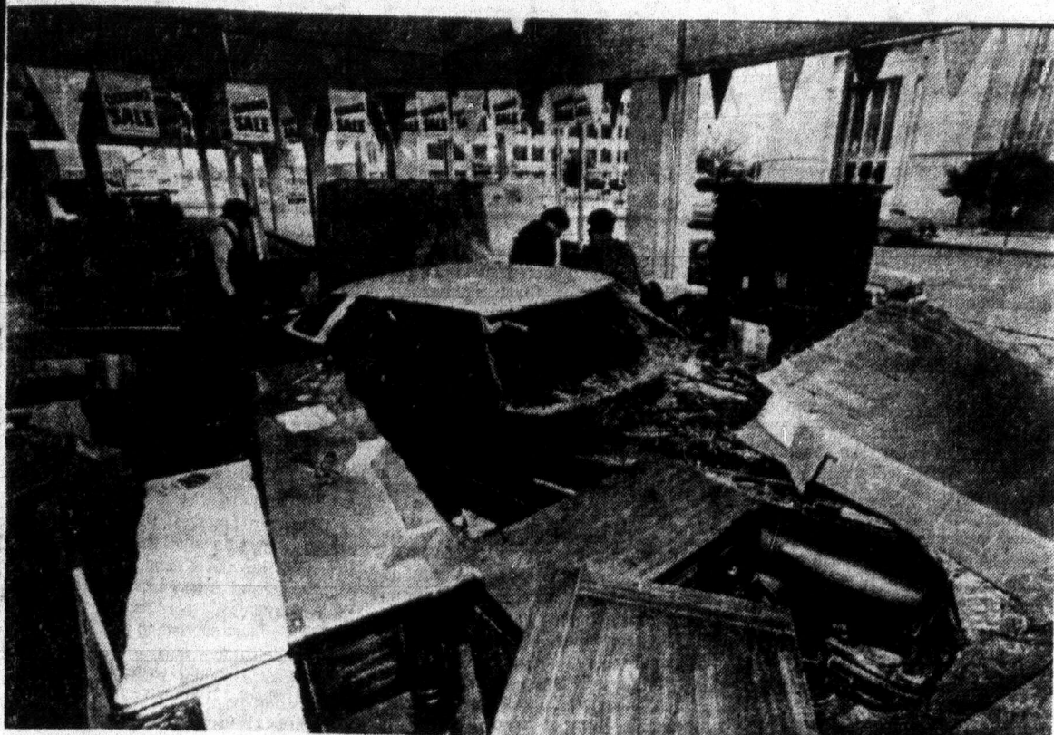
DRIVE-IN SERVICE? — This Sears and Roebuck in Wichita Falls received about $20,000 damage recently when a car drove through some plate glass windows at the pick-up department.
