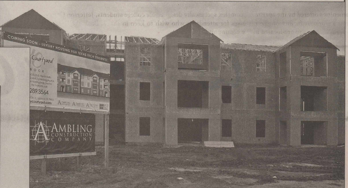
THE UNIVERSITY COURTYARD apartments are being constructed on Erskin Avenue, just west of Indiana Avenue. Once finished, the complex will offer several floor plans to satisfy the needs of college students. The apartments come fully-furnished and equipped with all major kitchen appliances.
