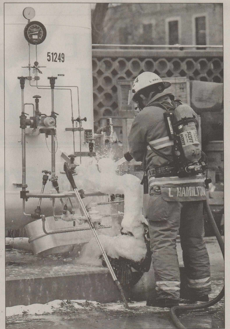
PHOTO BY KARL ANDERSON / The Daily Toreador LANCE HAMILTON, A lieutenant with the Lubbock Fire Department, uses water to hose down a tank of nitrogen which was reported to be leaking. When the department arrived, they found the tank was just emitting steam, which is normal.
