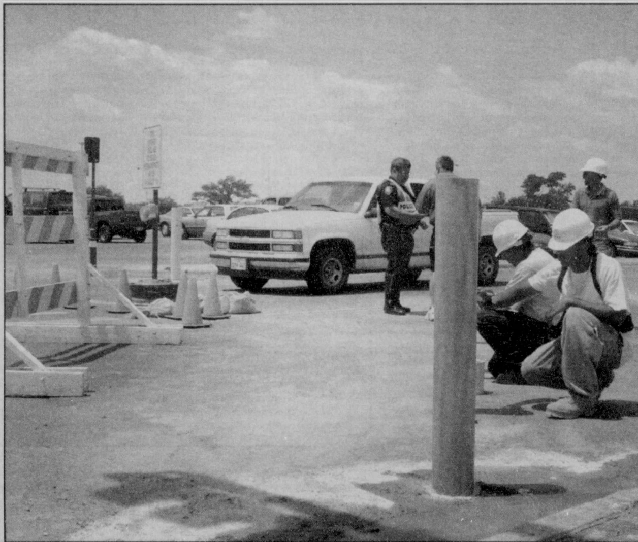
Construction workers from Lee Lewis Construction paint concrete and iron poles that will make up the road block for Red Raider Avenue. The avenue was permanently closed Tuesday, pending the renovations at Jones SBC Stadium. Joe Mays ■ The University Daily
