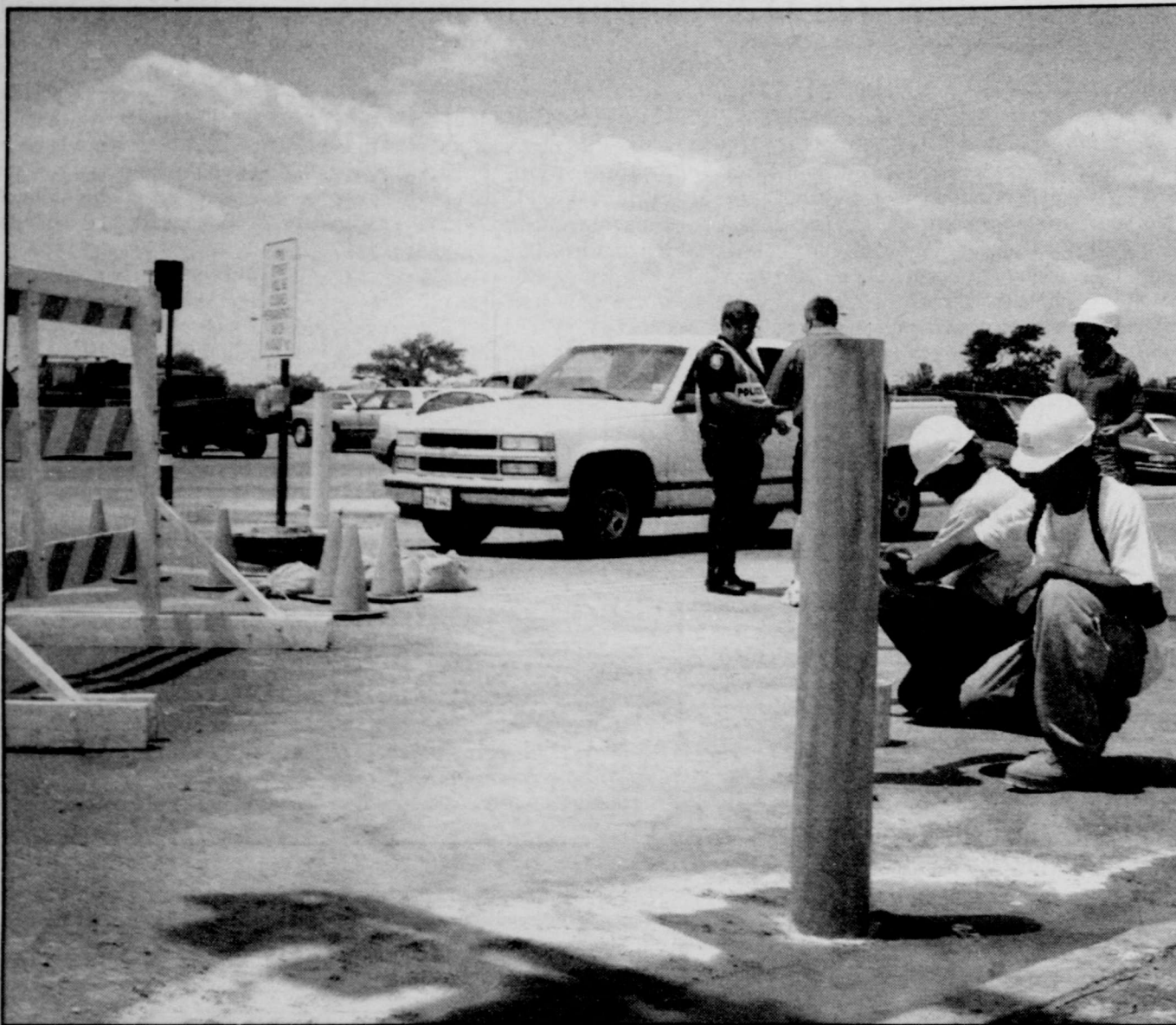
Construction workers from Lee Lewis Construction paint concrete and iron poles that will make up the road block for Red Raider Avenue. The avenue was permanently closed Tuesday, pending the renovations at Jones SBC Stadium.
