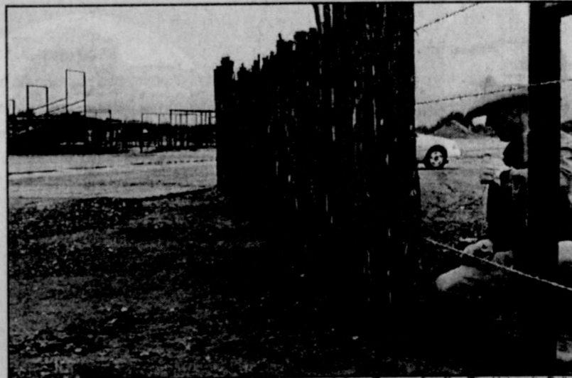
Jaime Tomas Aguilar/The University Daily Matt Buckner, a general studies major from Fort Smith, Kan., works on the gate to the entrance of Dub Park Arena on Tuesday. A donation to the arena has made numerous renovations possible.
