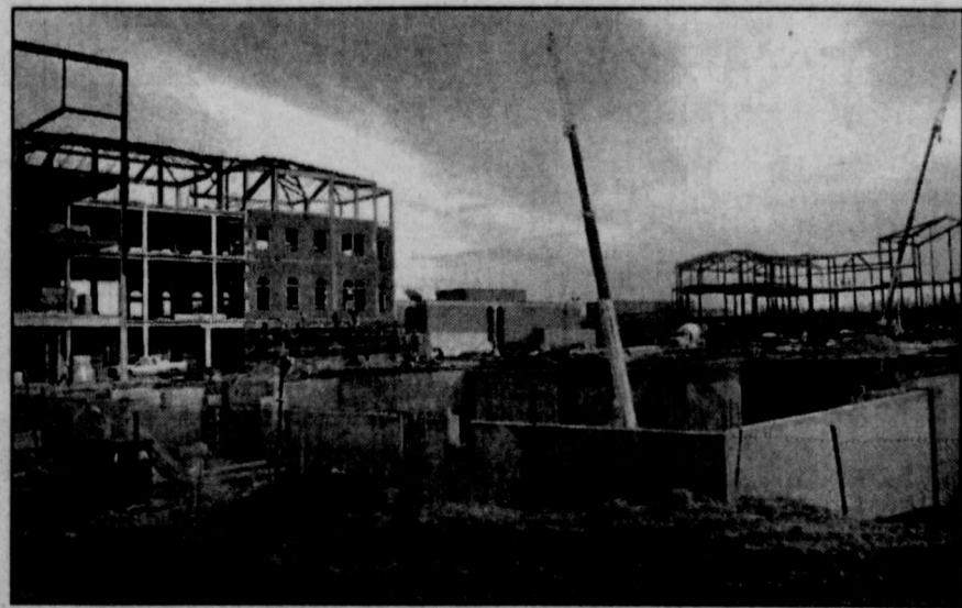
Construction on the English/Philosophy/Education Complex has progressed since this photo was taken in August.
