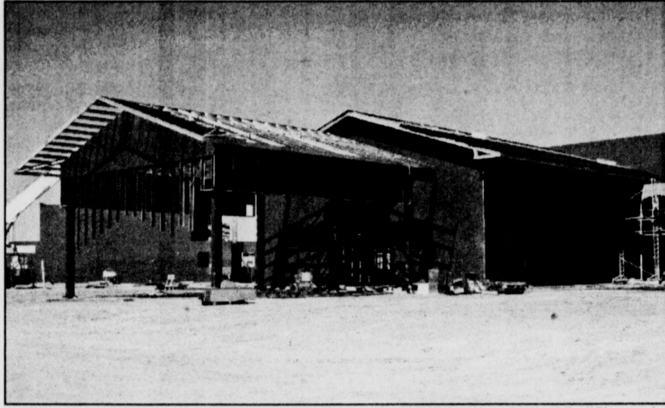
JAIME TOMAS AGUILAR/Staff Photographer THE GARRISON CENTER'S construction is in progress, one of several changes the Texas Tech Health Sciences Center will undergo during the 2001-02 academic year. The facility will serve as a geriatric care center where medical students can gain experience treating the elderly.
