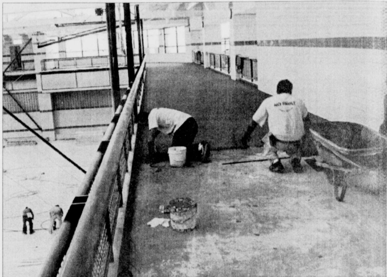
NEARING COMPLETION! Workers lay the material for the 1/8 mile elevated jogging track in the Robert H. Ewalt Student Recreation Center addition while workers below install the wood basketball floor.
