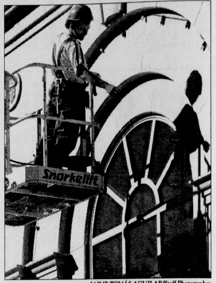
JAIME TOMÁS AGUILAR/Staff Photographer LEE GARCIA , A temporary worker from Labor Ready staffing agency examines his progress while hanging lights on West Hall Tuesday afternoon in preparation for the 44th annual Carol of Lights celebration to take place Dec. 6.
