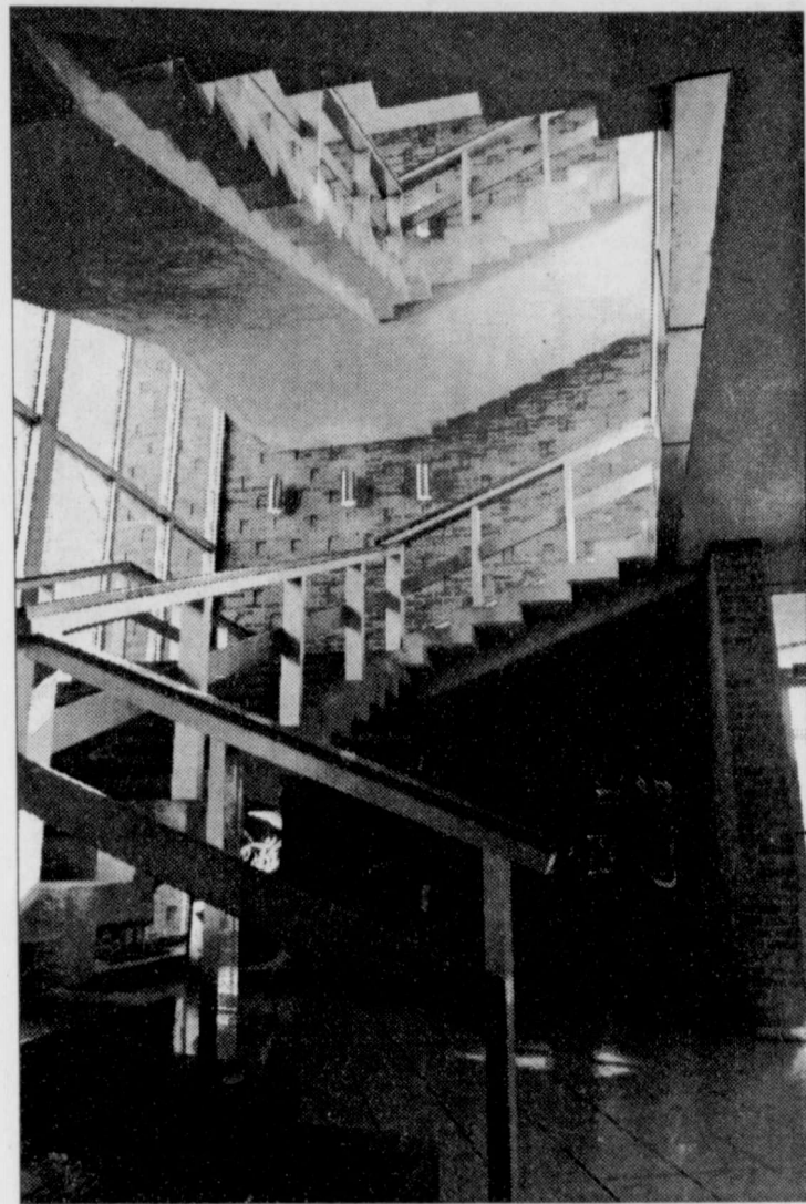
JAIME TOMAS AGUILAR/Staff Photographer THE OLD ENGLISH/Philosophy building is projected to be razed in a year and a half to meet fire code requirements.
