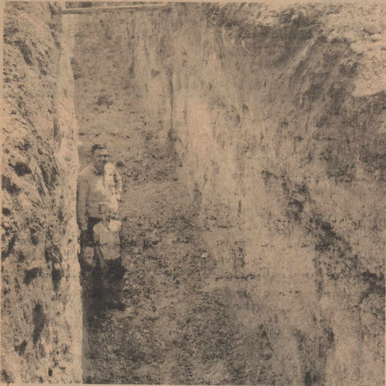
Dayton Elam and son, Paul stand in an opening ditch 10 to 12 feet deep. Note the line above their head. One of the problems of laying line through Gaines County is the depth the line has to be laid to clear other lines.
