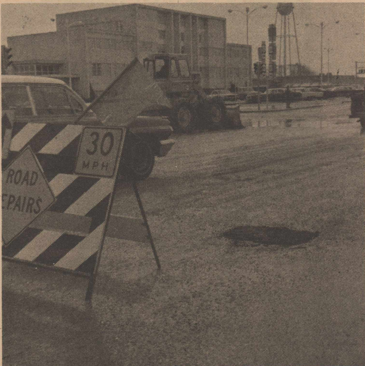
With more rain, ice, snow and freezes the Texas Highway Department has more and more repairs. Notice on the northwest corner of the courthouse, next to the bank, repairs are made each day for several days. Finally, on Monday they cemented in a block that they were having trouble with.
