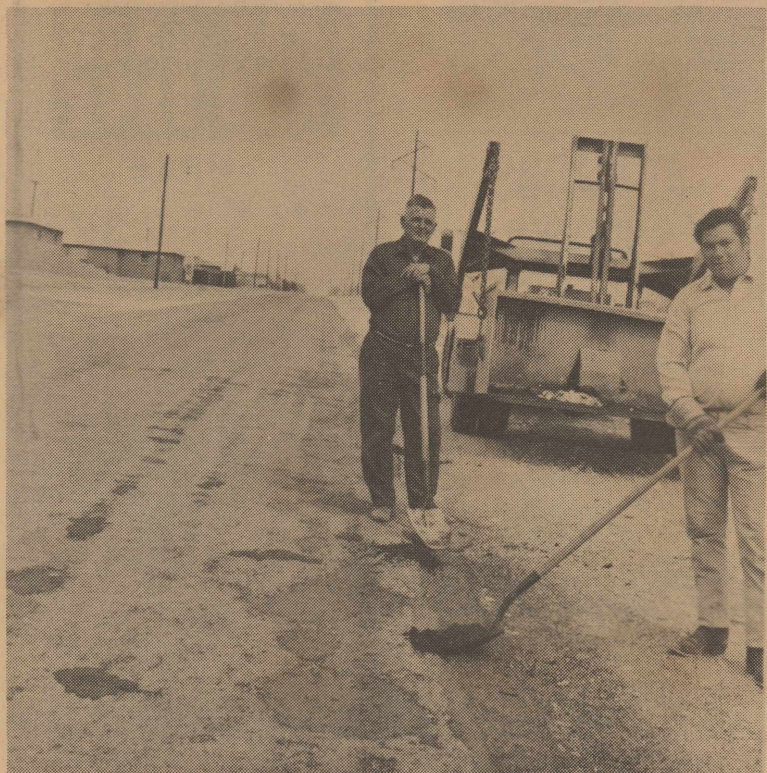
CITY EMPLOYEES ARE PATCHING SOUTH WEST AVE G. IT TAKES CONTINUOUS WORK TO KEEP OUR STREETS IN GOOD DRIVING CONDITION. IN THE FOREGROUND IS MIKE UBALLE AN EMPLOYEE OF THE CITY FOR FOUR YEARS AND ALTON STEVENSON HAS WORKED FOR THE CITY SEVEN YEARS.
