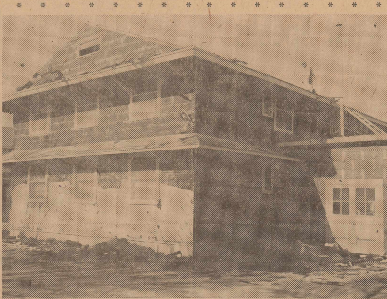
BEGAN SALVAGE.—Workers from a local school district began salvage Monday of one of the two-story temporary buildings in the 220 block to make way for construction of two new permanent type dormitories. Construction on the new buildings is expected to begin sometime in February. Photo by Roco
