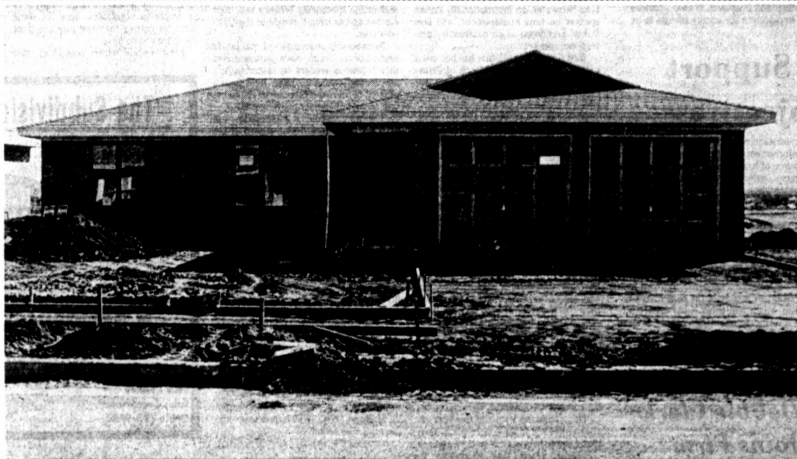
UNDER CONSTRUCTION—This home in South Lubbock is nearing completion along with a final phase of activity in the Potomac Park addition. The Potomac Park area was started in 1972 and now has 475 homes completed out of an original 489 sites for single-family homes. This house, built by Edwin Roberts, is at 8415 Elkridge. Six
