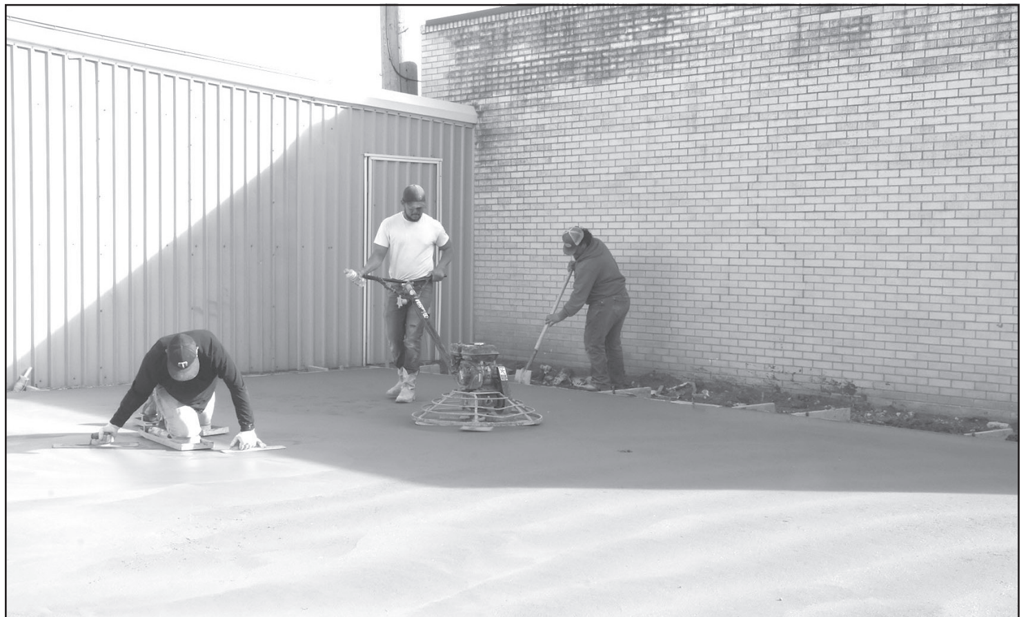
Work on the new Friends of the Public Library Bookshop is underway. Trejo's Roofing & Construction finished the concrete padding this past week.
