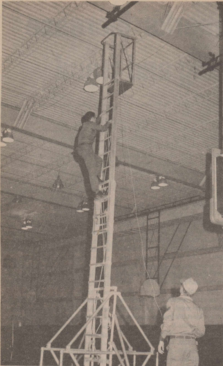
SrA. Robert D. Van Velac (on ladder) and SrA. James L. Carter install new cables and replacement speakers for the base gym in preparation for the annual Christmas Classic basketball tournament. Comm Squadron personnel will be on hand throughout the event to ensure the new equipment operates smoothly. (U.S. Air Force Photo)
