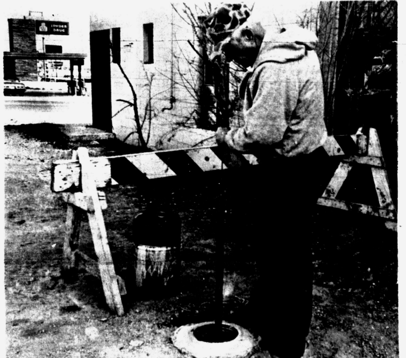
WELL TESTING — City employee Kenneth Rinehart pulls up a tube from the test well behind the former Texaco station at the southwest corner of 37th St. and College Ave. The city has been bailing varying levels of gasoline from the well since Feb. 21. (SDN Staff Photo)
