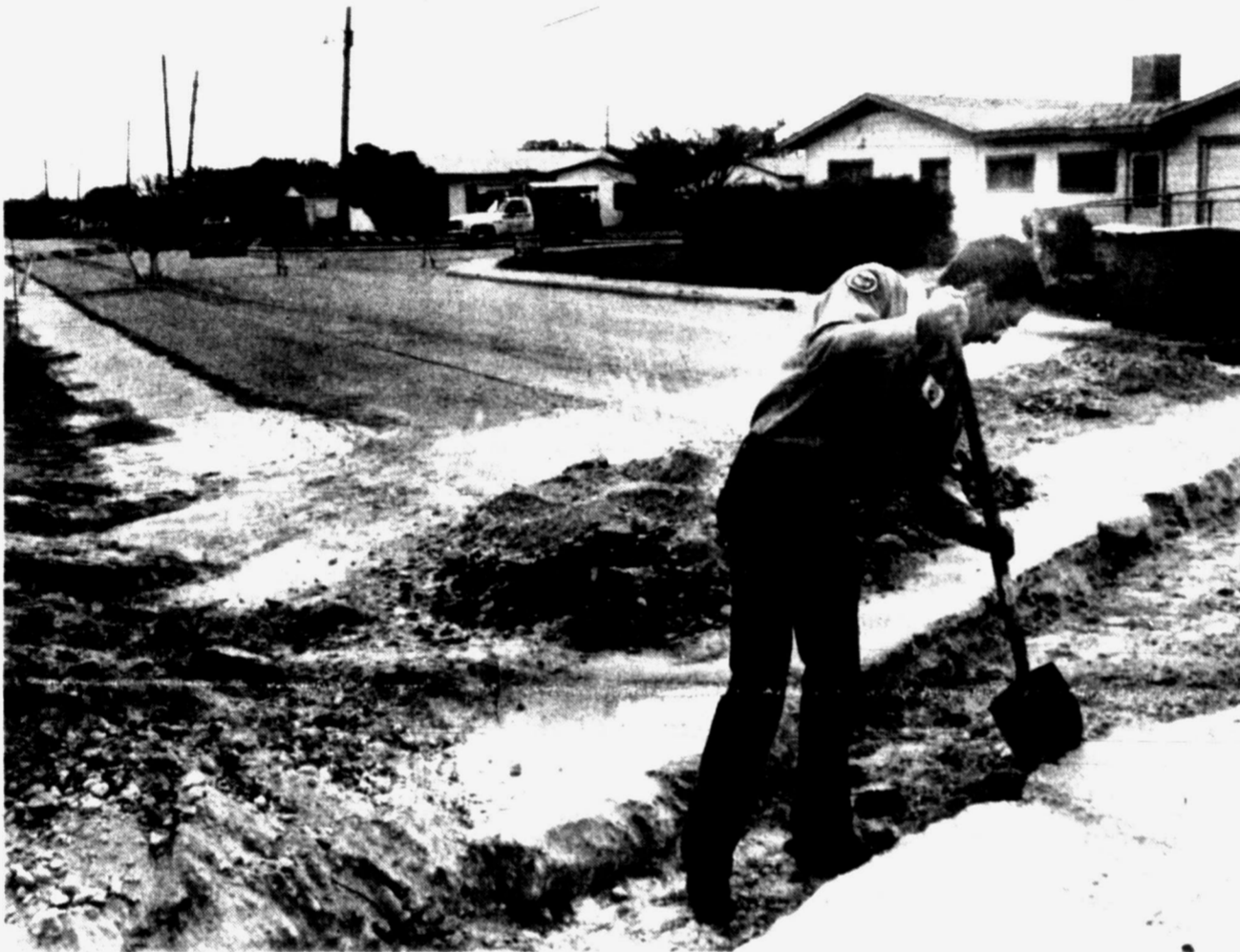
37TH STREET WORK — A city crew has been burying conducting lines along 37th Street in preparation for the street's widening project. Earlier this week, the State Department of
