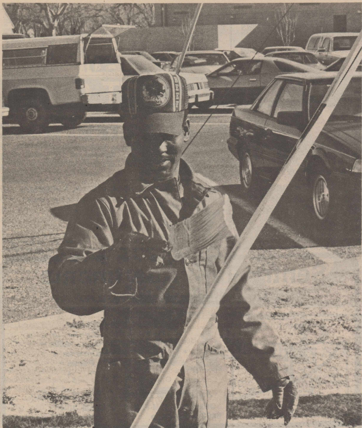
A1C Jerry Green of the 64th Civil Engineering Squadron paints a telephone pole guy wire guard. Airman Green works with the Exterior Electric Shop of CES.
