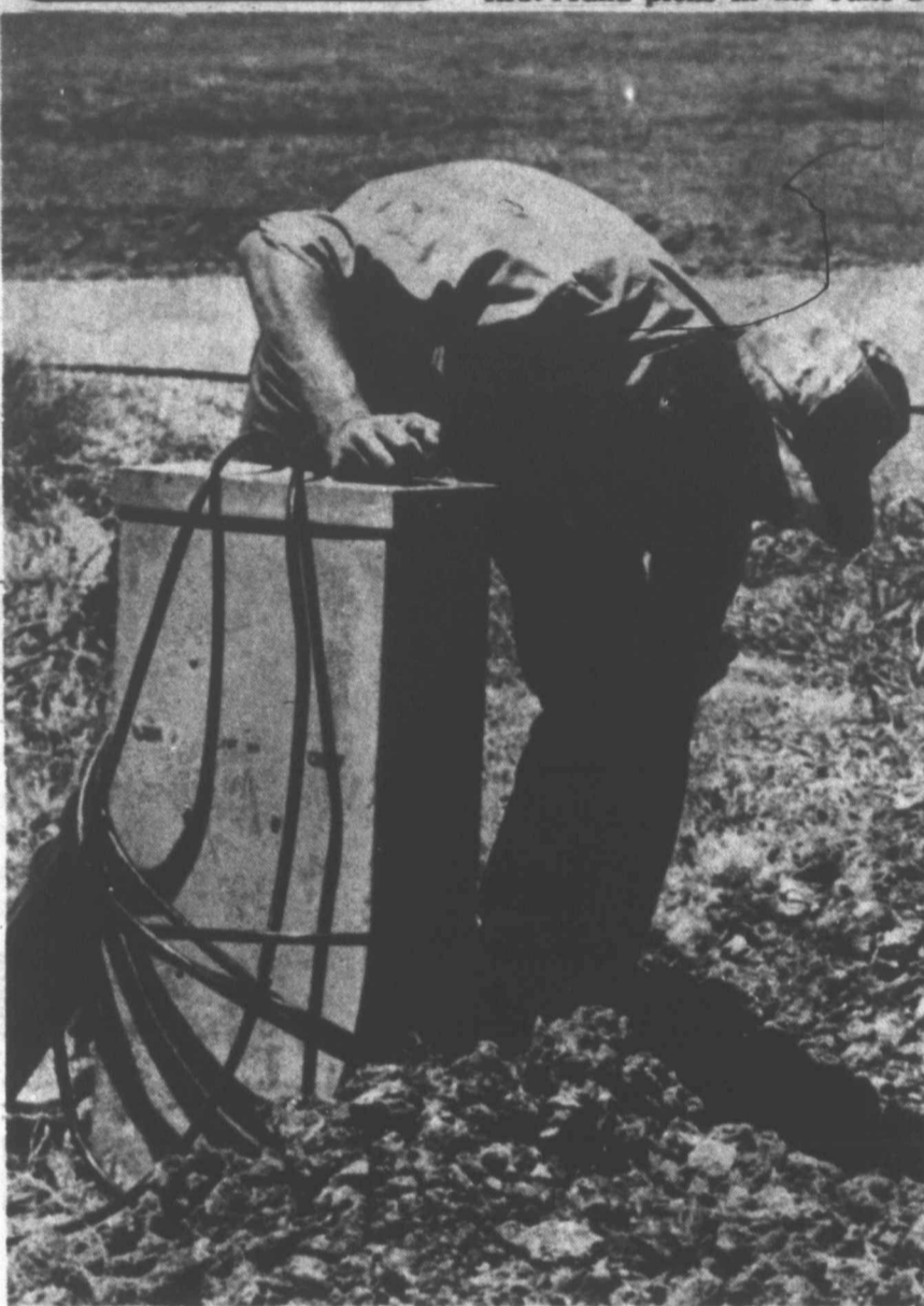
GOLF COURSE MAINTENANCE — Carl Stewart is among the maintenance personnel at Western Texas Golf Course working on repairing electric lines to the course's underground sprinkler system. According to pro shop manager Dave Foster, the facility will remain open during the work which is scheduled to be completed in August. (SDN Staff Photo)
