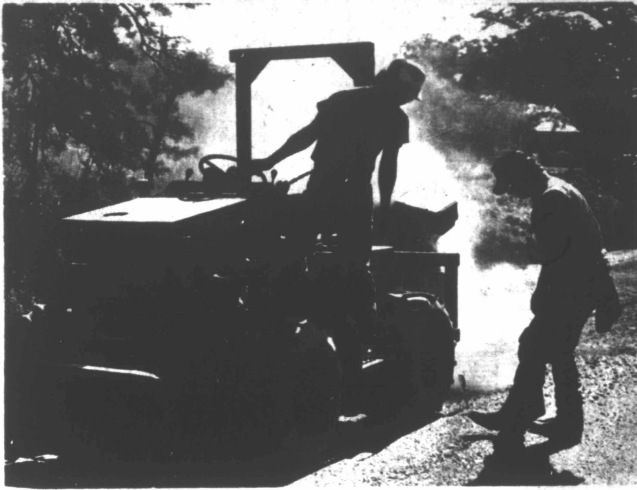
37TH STREET WORK — Johnny Garcia and Paul Villaneuva work along 37th St. The effort is ongoing to replace a water line beneath the street, prior to the scheduled widening of 37th from College Ave. to El Paso. (Howard Bigham Photo)
