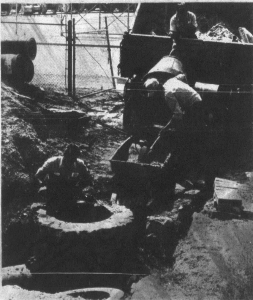
PUMP INSTALLATION — Employees at Snyder's Water Pump and Filter Plant recently replaced a water pump and repaired a collapsed drain which had caused some flooding in the pump room. Those pictured are Darrell Boone, in the ditch, and Gary Sharp and Juan Becerra, in the truck. (SDN Staff Photo)
