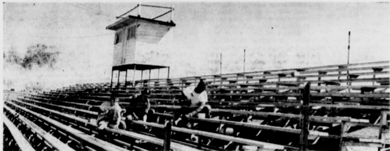
TAKING SHAPE —Stanton High School coach Harlin Dauphin, right, and two of his football players, Arnold Fincher, left, and Jerry Polson, install seats in the new bleachers at Buffalo Stadium. When completed, the north and south stands will accommodate 3,000 persons.
