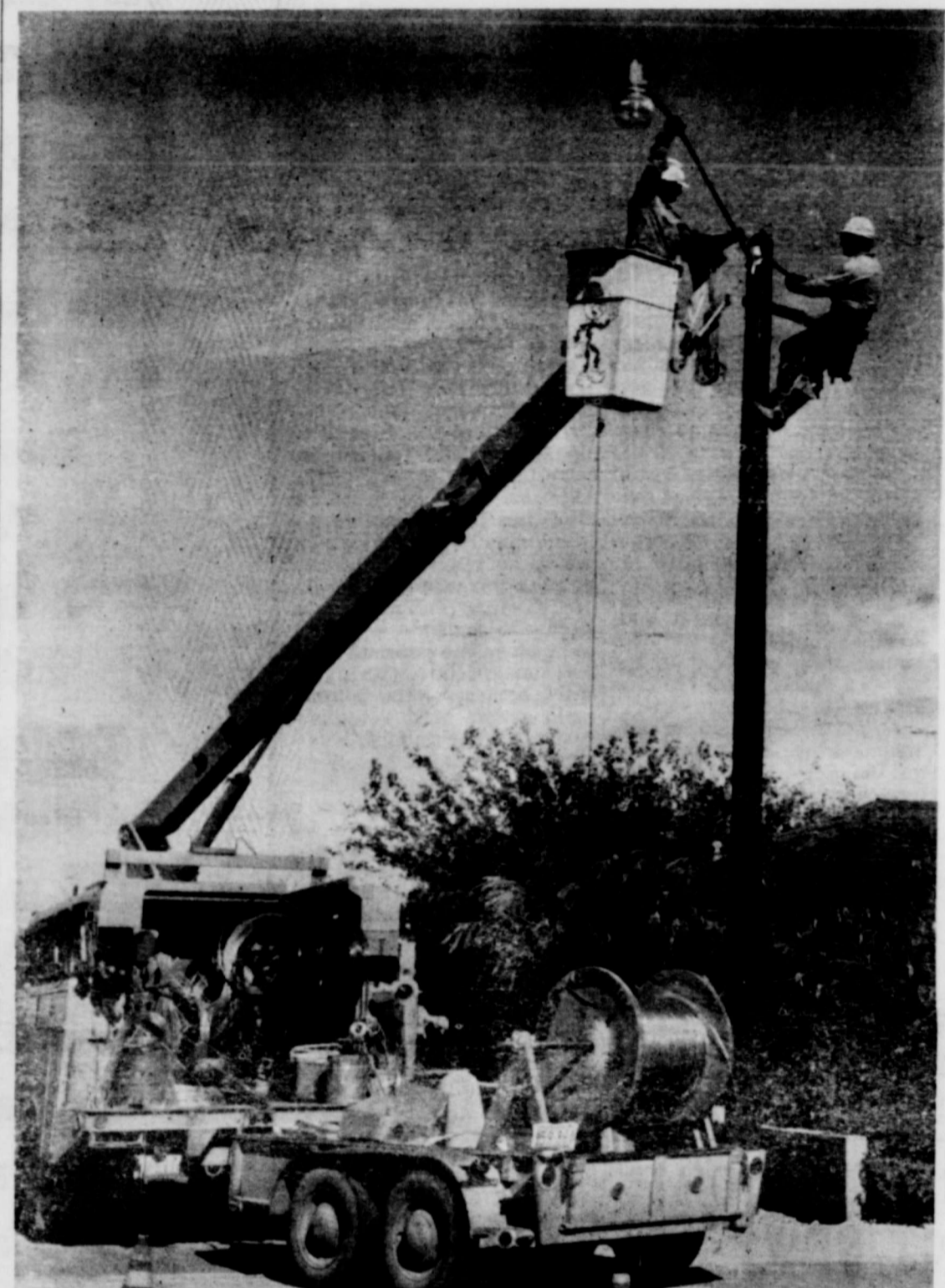
BRIGHTER CITY—The city officials have ordered the installation of 92 mercury vapor lights. The program promises to make Stanton a well lighted city in the business and residential areas. The photo above shows workers of Texas Electric Service Company in installation action. All the lights will be installed by the end of December.
